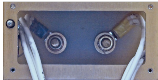
Figure 2-11 HV Output Cables Secured to Studs inside FPS
