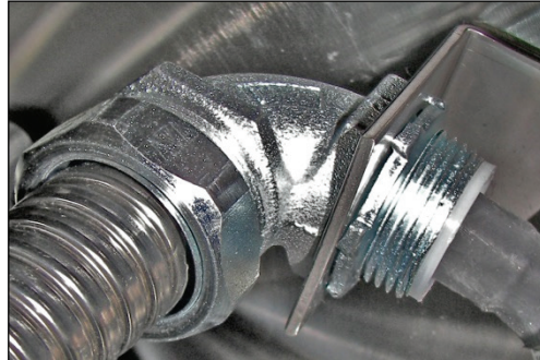
Figure 2-14 HV Conduit Properly Secured to Bracket
