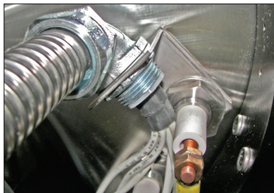
Figure 2-13 HV Conduit Bracket Properly Installed on HV Feedthrough
